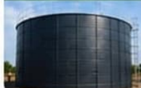
MS / STEEL FIRE WATER TANKS
